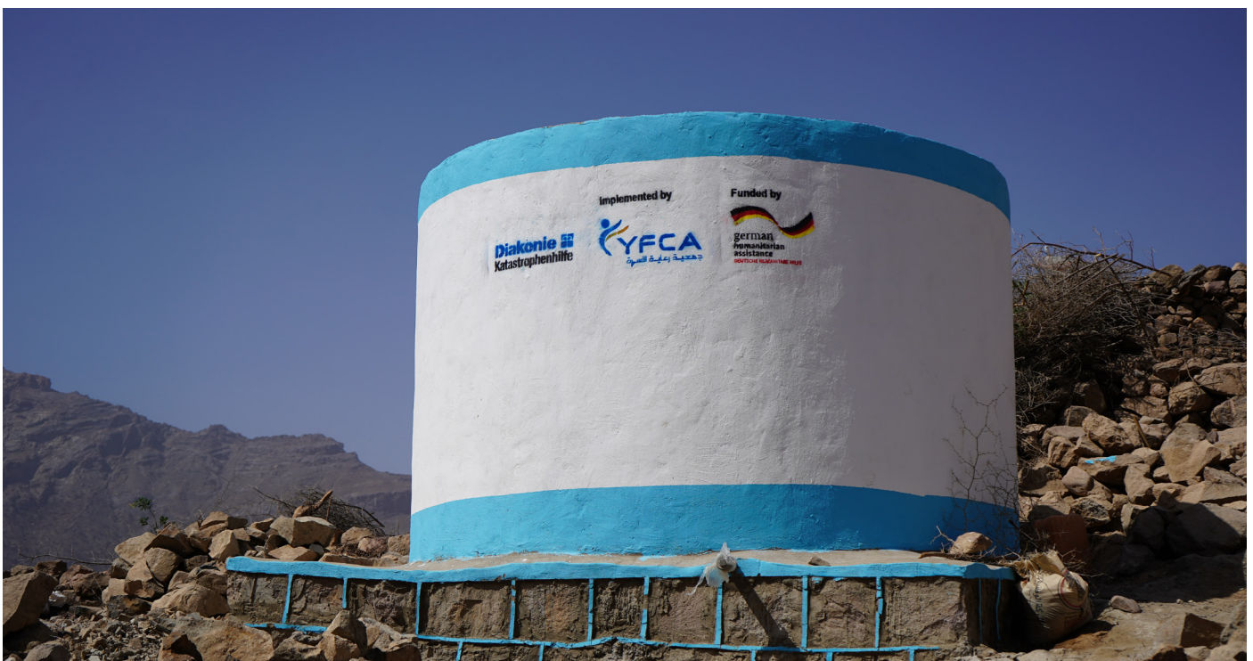
One of the 26 constructed water tanks in Al Aawkima area.
