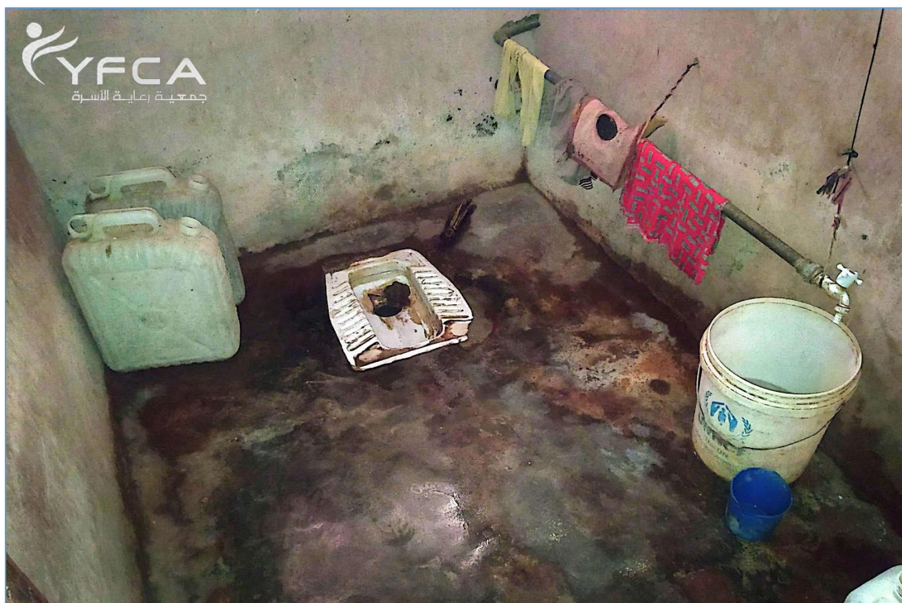
Photo 11 One Type of HH Latrine _ Khanfar District
