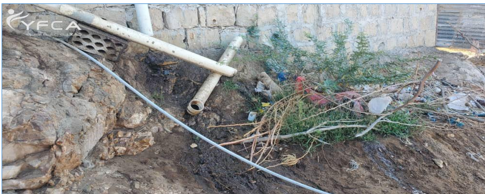
Photo 14 Sewage Flowing into the Streets, Khanfar District
